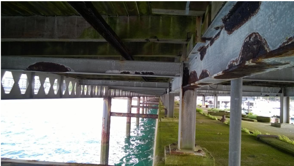
10 View of failing galvanised protection to steel frame below boardwalk between theatre promenade and widening
