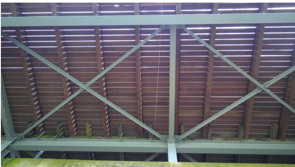
11 View under boardwalk showing recent timber decking installation over 1970s-installed galvanised frame refurbished with protective coating
