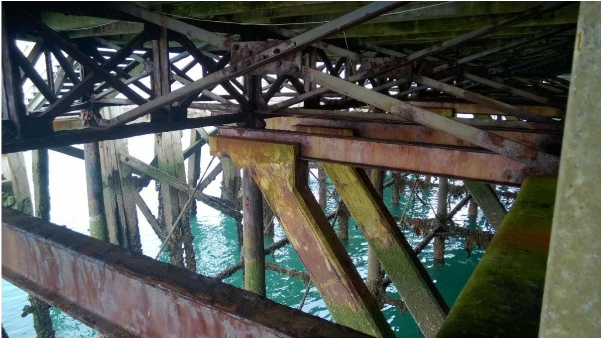
6 General view below pier head widening showing corrosion to steel framing and significant spalling (cracking) of concrete encased props
