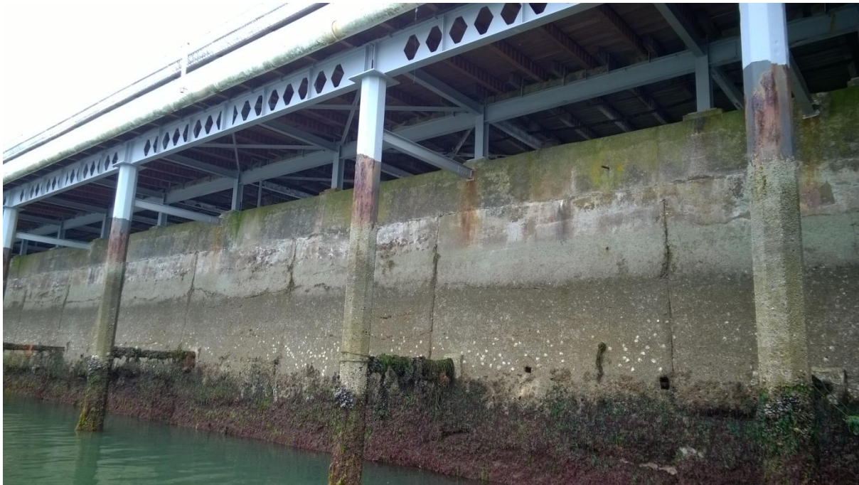
2 1970s-installed galvanised steel frame below timber boardwalk supported on the original concrete and masonry pier, and by steel piles (columns)
