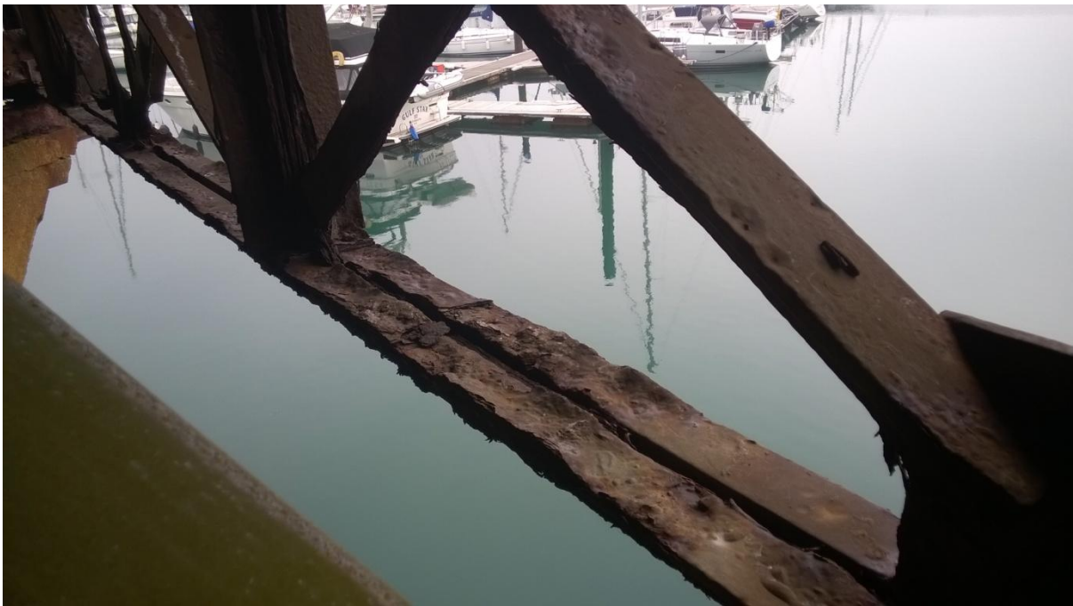
7 Heavy corrosion to pier head steel lattice
