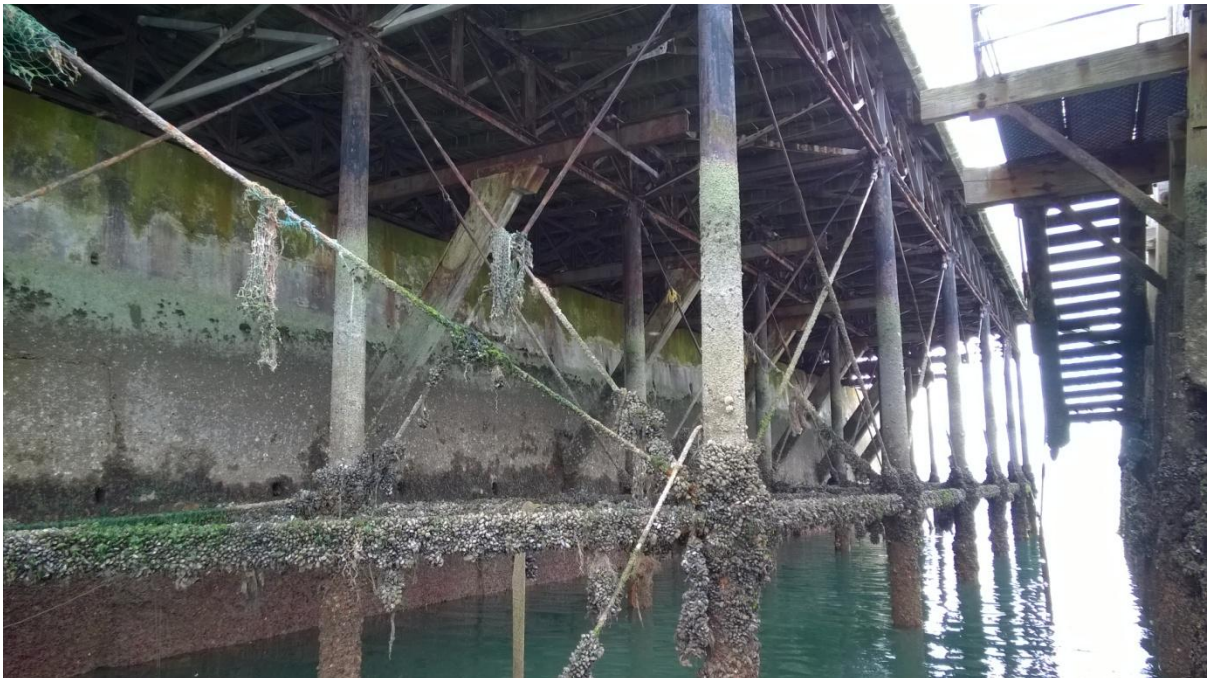
5 Piled support to boardwalk widening showing failure of diagonal ties. The piles supporting the lattice framing have suffered accelerated low water corrosion (ALWC) and are severely corroded, having lost an average 1mm section thickness per year. The timber landing is to the right of the picture
