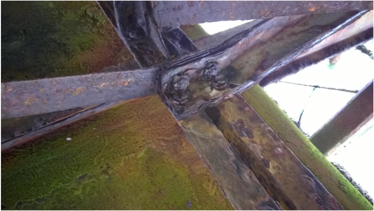
8 Heavy corrosion to pier head steel lattice, showing delamination over residual steel section
