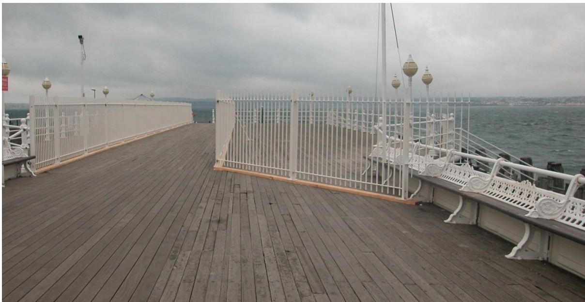
3 Widening at the pier head; fencing installed in 2007 to close unsafe areas, thoroughfare maintained for public access to pier beyond
